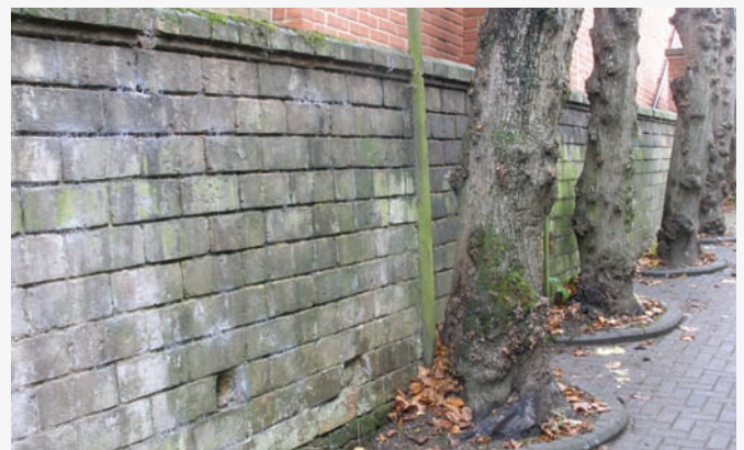
Wall constructed in patent Hitch bricks, in the lane behind No 66 High Street.
