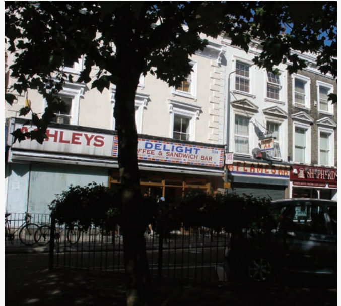
No 33 High Street (to left) Handsomely proportioned Mid Victorian late Classical town house, slightly obscured by later shop fascias.
