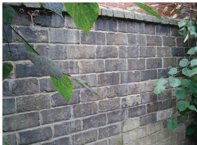
Fig.8: Caleb Hitch's patent brick walling to the alley linking High Street to Legra Avenue – an important survival of considerable local and possibly national significance.
