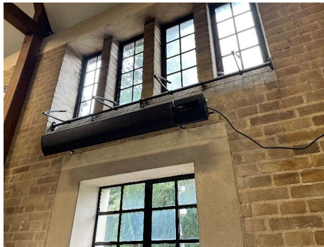
Figure 37: Wall mounted radiant tube heaters
