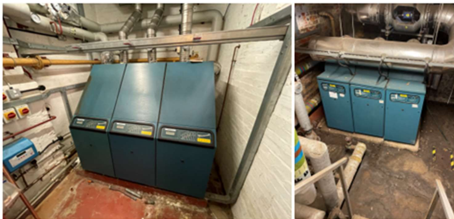
Figure 28: Gas boilers at the east end of the Old Building (left) and the basement plant room at Spanish Ambassadors House (right)
