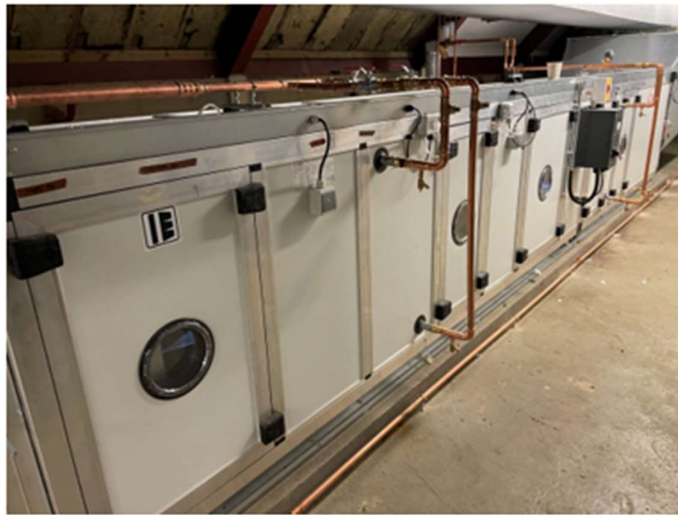
Figure 21: The New AHU 1 supply section serving Level 2 council offices
