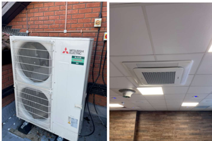
Figure 14: A/C outdoor unit (left) and indoor unit (right)
