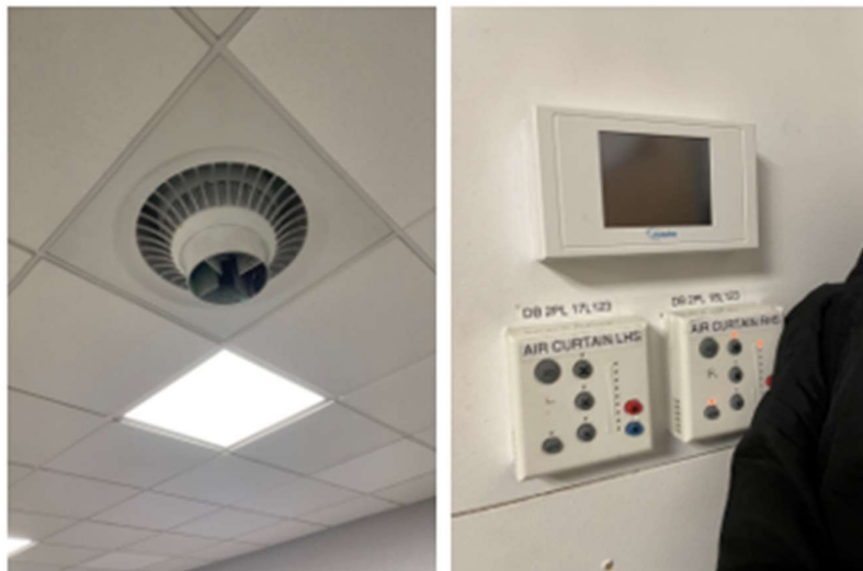
Figure 17: Local vent unit (left) and Nuairé controller (right)
