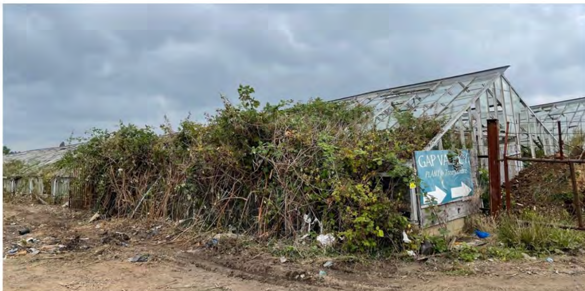
View of main glass houses within the site which are currently being demolished
