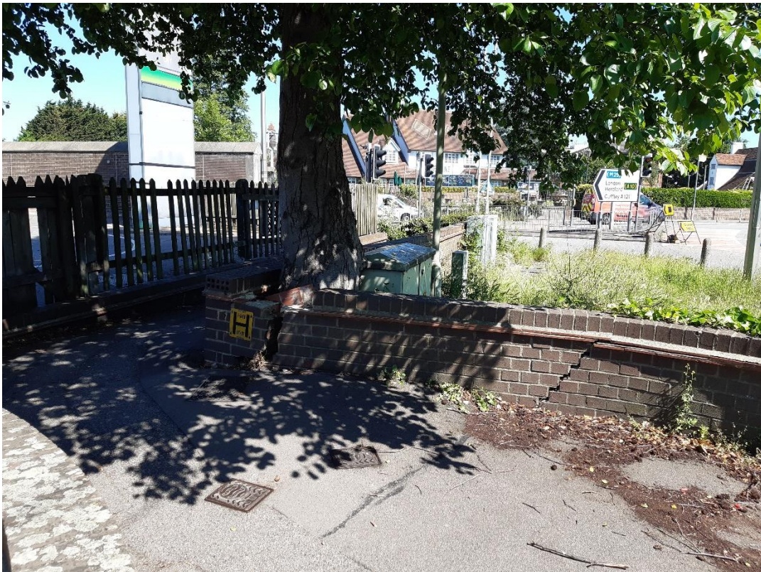
Footpath boundary wall damage
