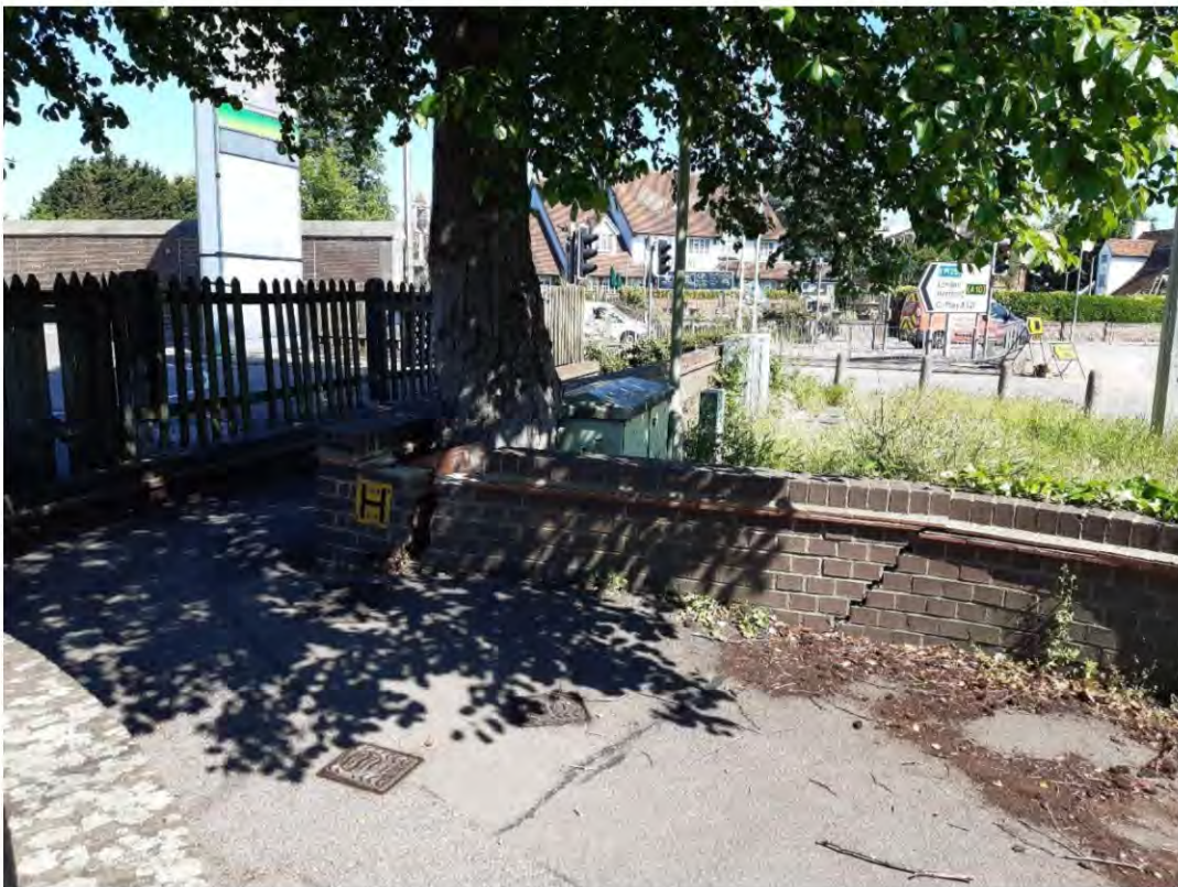
Footpath boundary wall damage
