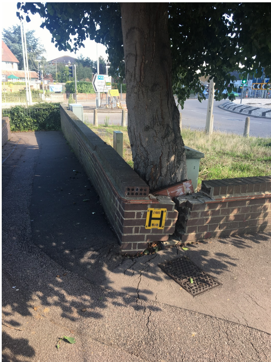
Photo 2 – T1 (illustrating existing damage to retaining structure to site-side base)
